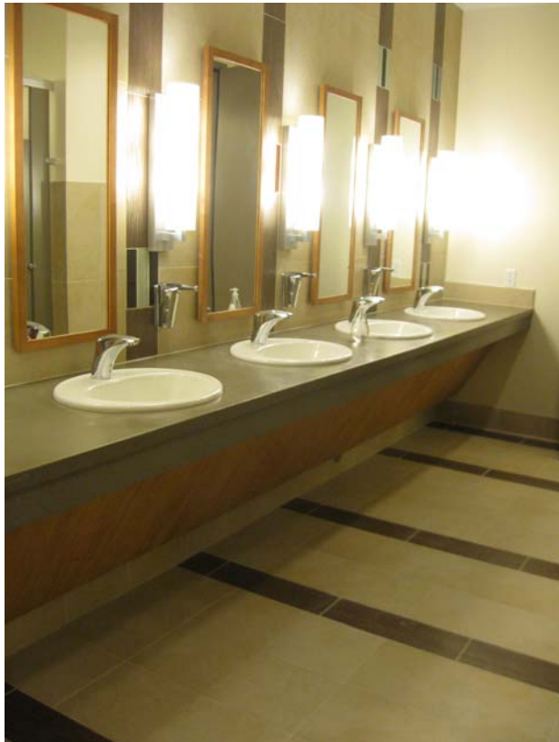
Plumbing fixtures in the restroom cut water use in half
