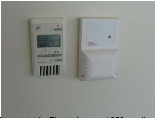
Thermostat for Thermafuser and CO2 monitor
