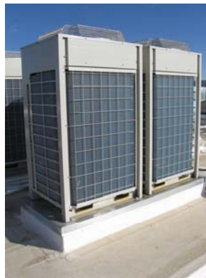
Daikin system on roof
