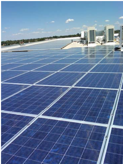
90% of the PV power is generated on the roof
