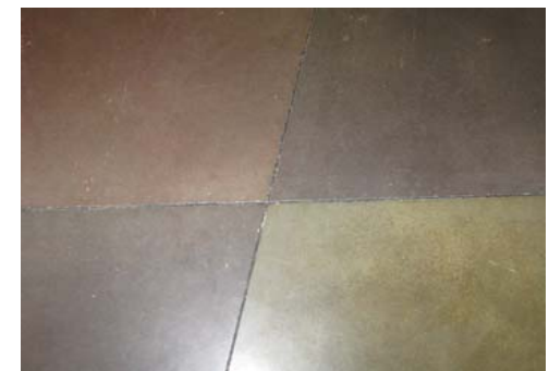
Stained concrete flooring
