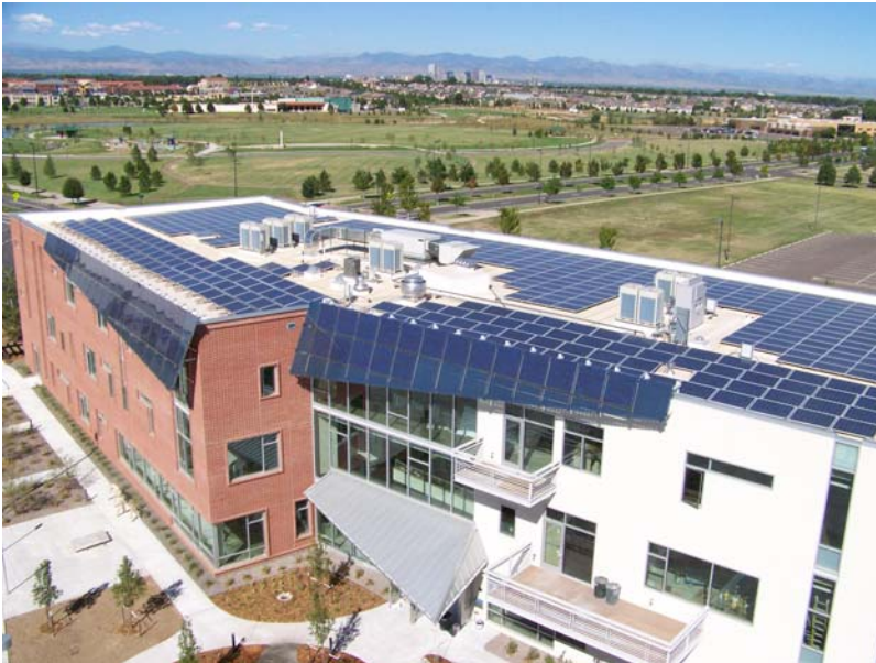
410 Sunpower PV panels
